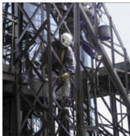
A 15-month painting project, involving 60 tonnes of paint and 25 workers, is all logged in the CMMS
